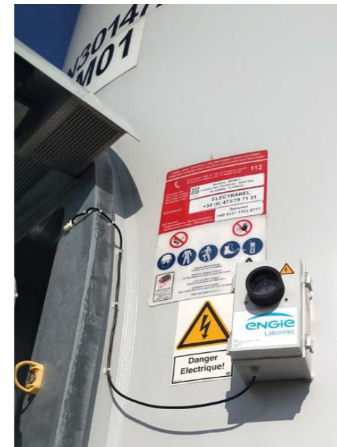
The ultrasonic detector at the turbine base
