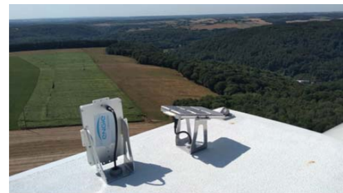
NRG deterrent speakers fixed to nacelle
